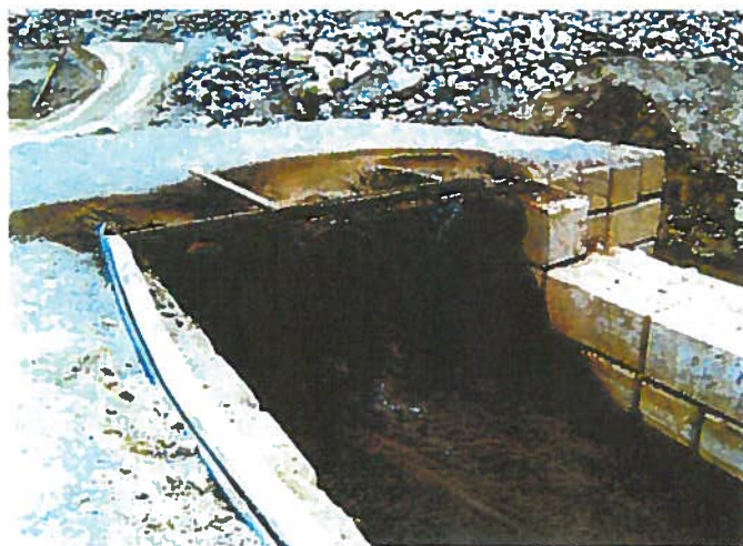
Following the addition of the flocculent solutions, a three outlet manifold discharges the treated water into the rectangular floc-sand pond.
