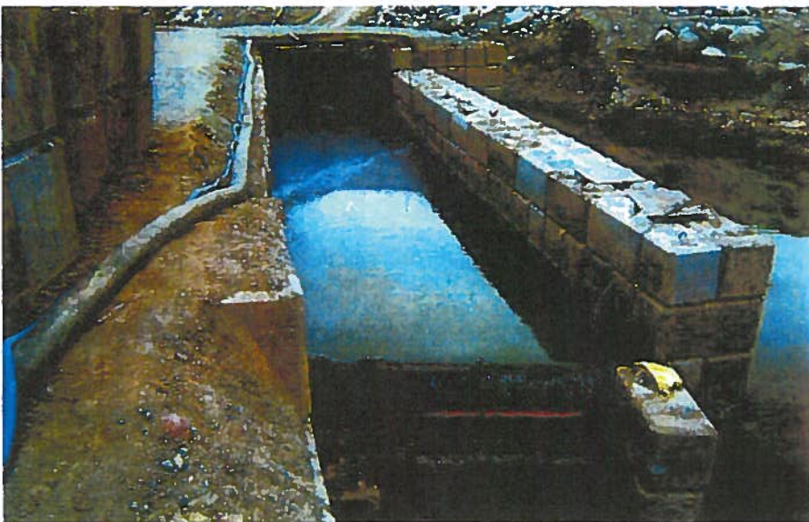
Treated water discharges into a rectangular 18.3 m x 4.6 m x 1.5 m floc-sand pond.
